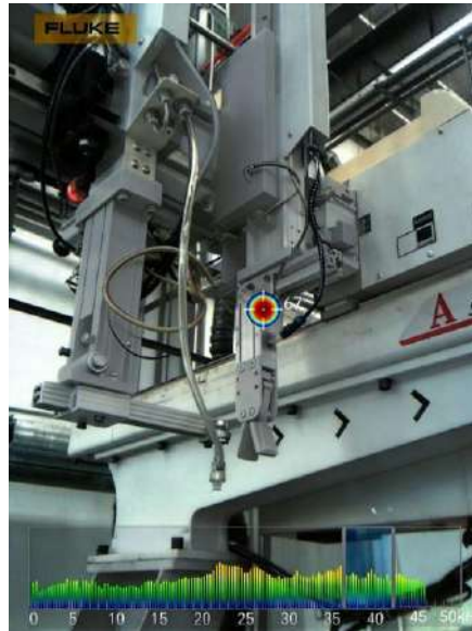
Compressed air leak detection of injection molding machines
